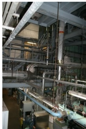
Pacific West Biomass Conference & Trade Show tour attendees saw a maze of pipes, valves and gauges during a tour of Seattle Steam which distributes steam to more than 200 downtown buildings.
